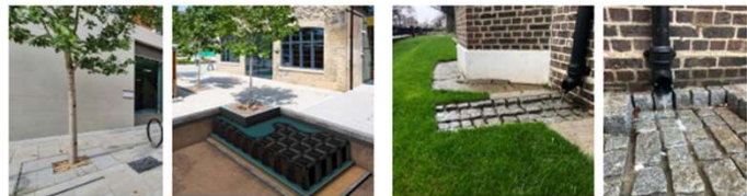
5 Engineered tree pits that manage rain water run off and benefit longterm tree health.
